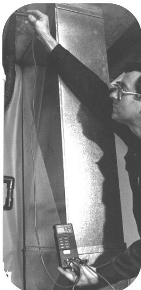
FIGURE 62 TEMPERATURE RISE MEASUREMENT
