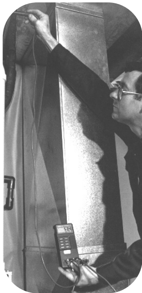
FIGURE 48 TEMPERATURE RISE MEASUREMENT
