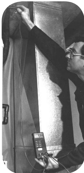
FIGURE 50 TEMPERATURE RISE MEASUREMENT
